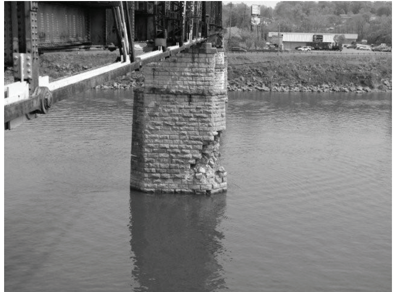
Damaged bridge pier on RJ Corman's Memphis Line at Clarksville, TN. Repairs are underway. (Submitted by Chris Dees, photographer unknown)
